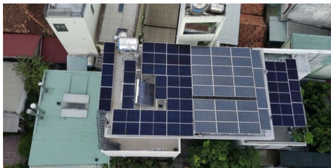
Solar Hybrid 28,83 kWp
